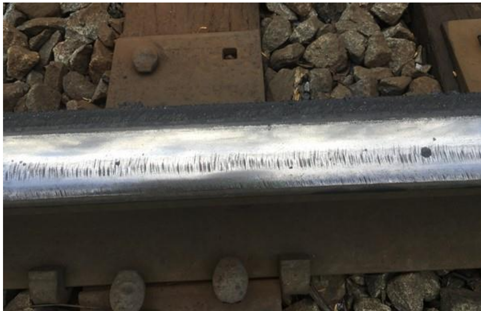
Figure 5-5: Picture from field survey of the right hand rail near MP 0.4. Heavy TORFM can be seen on the field (outside) side of the rail. Heavy grinding marks can be seen on the gage (inside) side of the rail.
