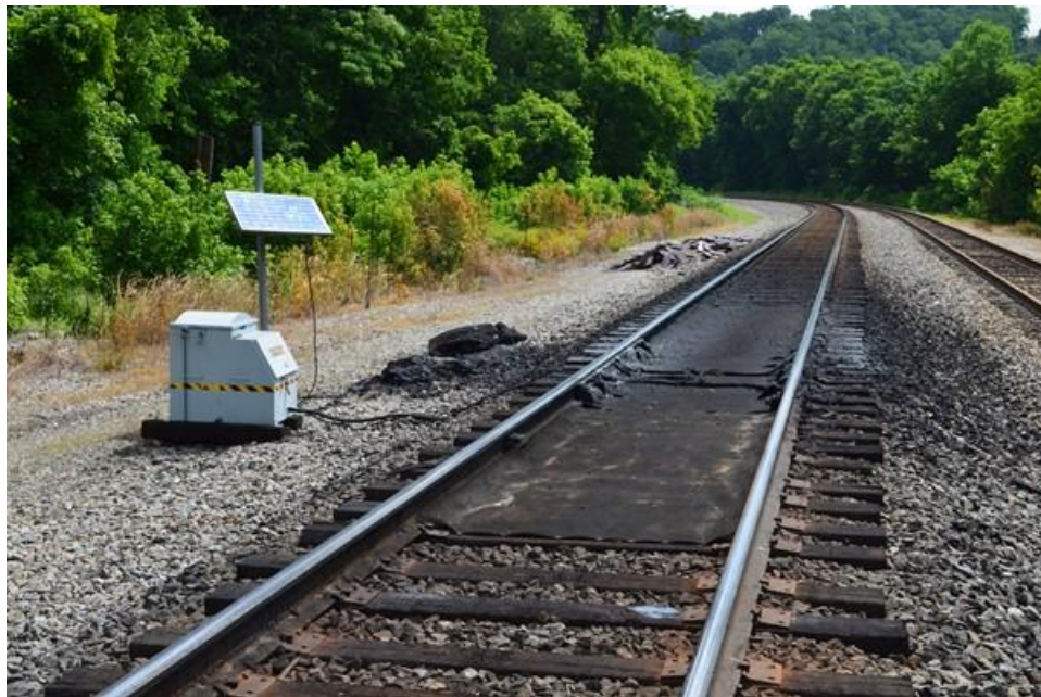
Figure 1-1: A gage face wayside applicator applies flange grease to the gage corner of the rail and the wheel flanges of passing wheels.
