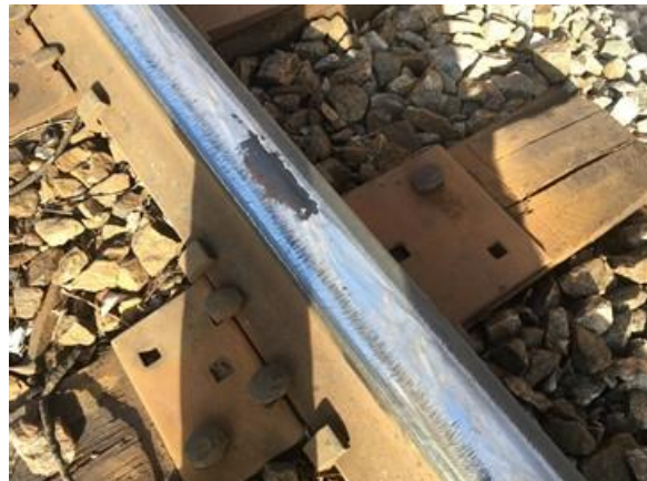
Figure 5-19: A crushed leaf can be seen packed onto the surface of the rail
