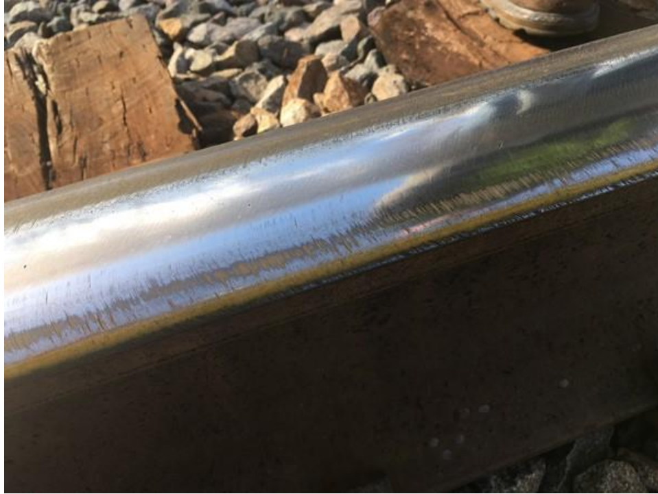
Figure 5-16: A field survey of the track near MP 3.7 shows limited signs of TORFM
