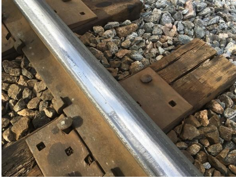
Figure 5-12: Patchy TORFM condition in a sharp left hand curve
