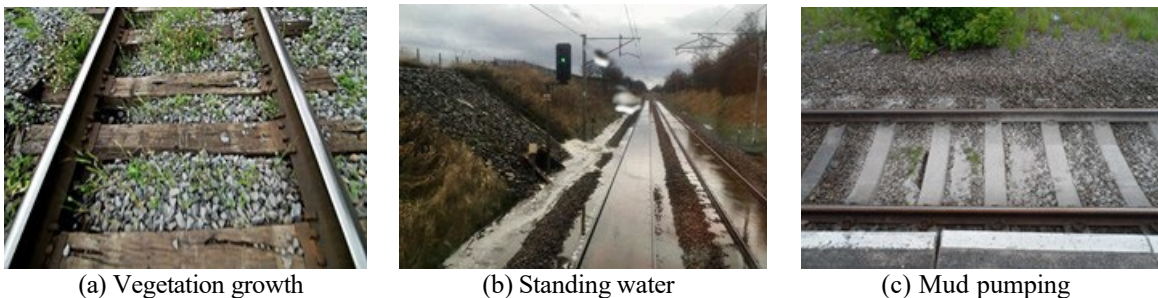
Figure 2.2: Rail Track Anomalies
