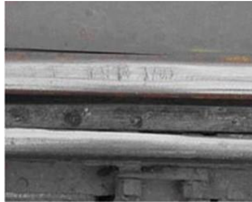
Thermal cracks on burned stock railhead
