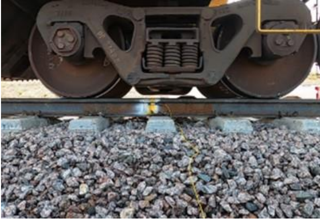
Welding defect 1: 0.8 in x 0.6 in. Location: 0.7 inches below the surface
