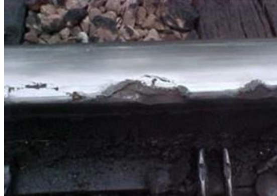
Side shells corrosion
