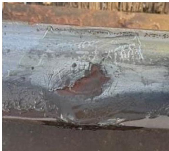
Surface defect: 1.2 in * 0.5 in
