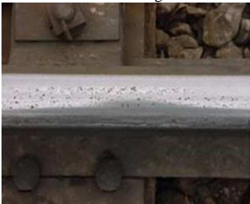
Flaking caused by centralized loading
