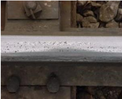
Flaking caused by centralized loading
