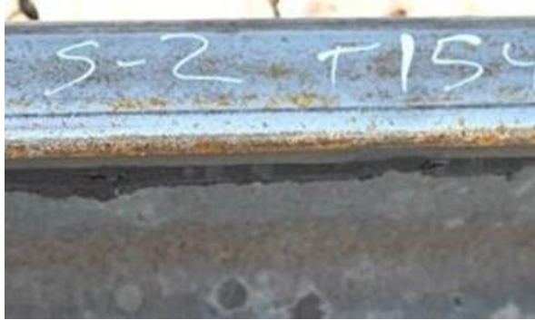
Figure 22 Rail crack in the web
