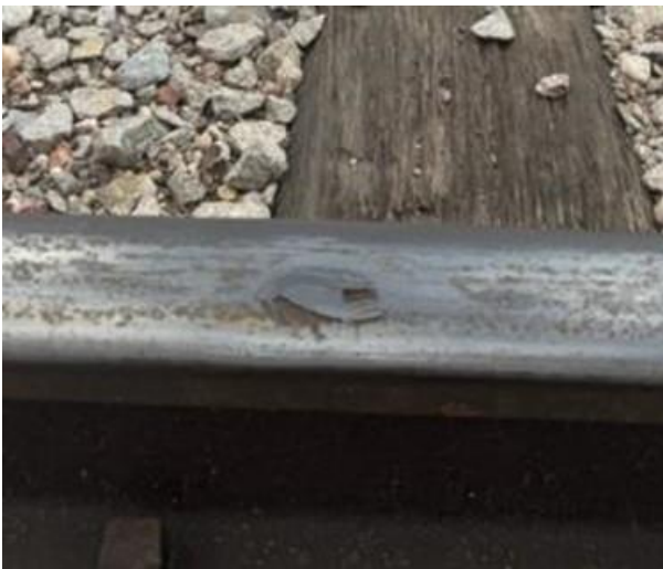
Surface defect: 1.3 in * 0.7 in
