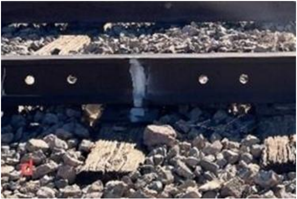
Welding defect: 0.2 in * 0.3 in. Location: 2.5 inches below the surface
