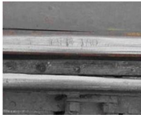
Thermal cracks on burned stock railhead
