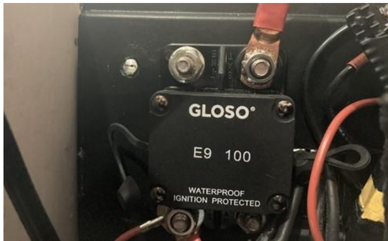
Figure 0-3: Installation of the auto-reset circuit breaker
